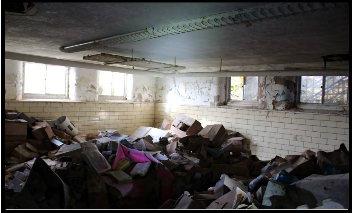
11 Another room in which the light fixtures could not be reached.
