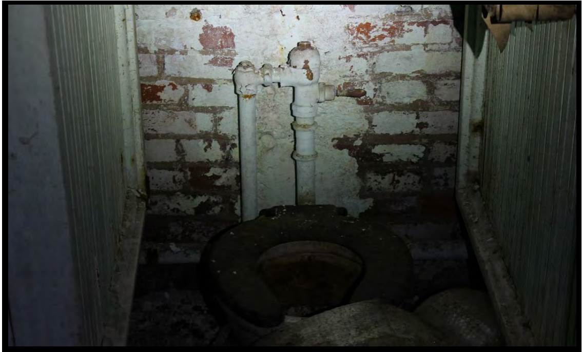
13 Galvanized piping was seen in the basement. No lead solder was observed.
