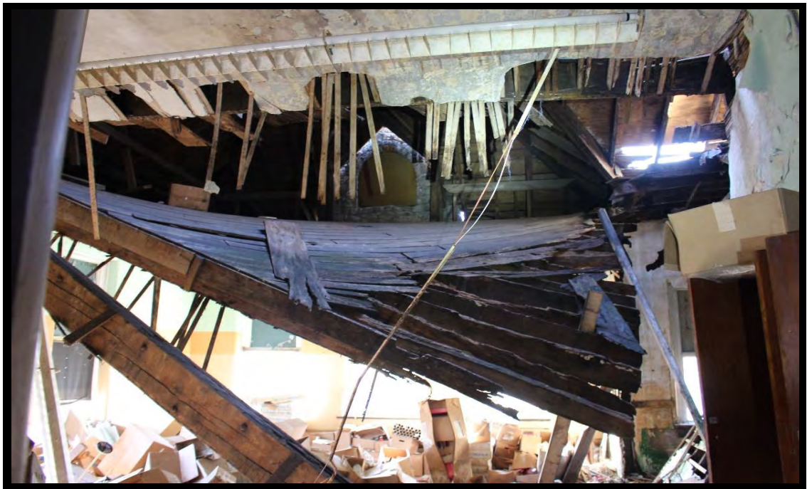
14 Another collapsed room.
