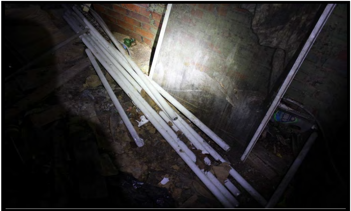
12 Some florescent light bulbs scattered in the basement.
