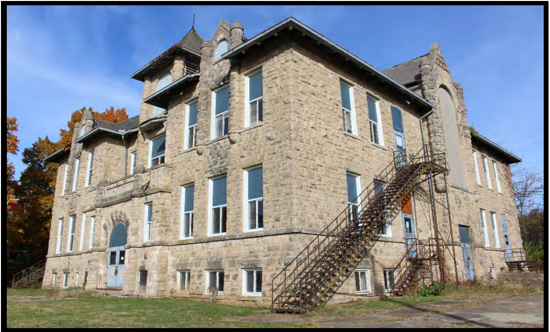
2 This is a two-story stone building with a full basement. The southeast corner of the building.
